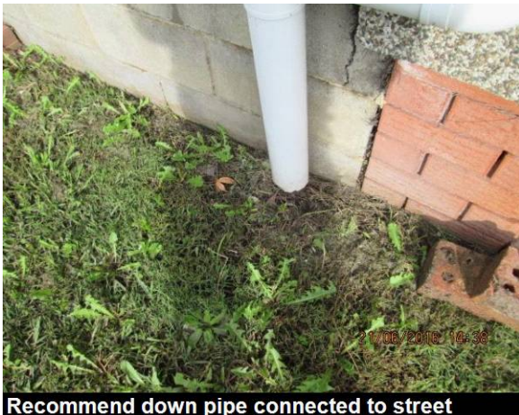
Recommend down pipe connected to street
