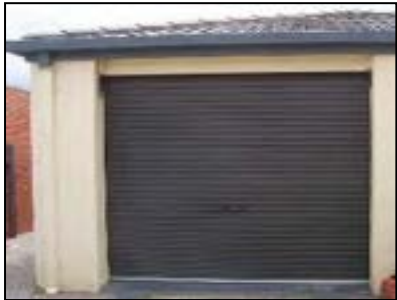
NON-COMPLIANT ROLLER DOOR
