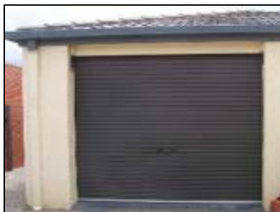
NON-COMPLIANT ROLLER DOOR
