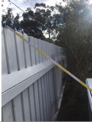
Example of 60 degree wedge on fence rails
