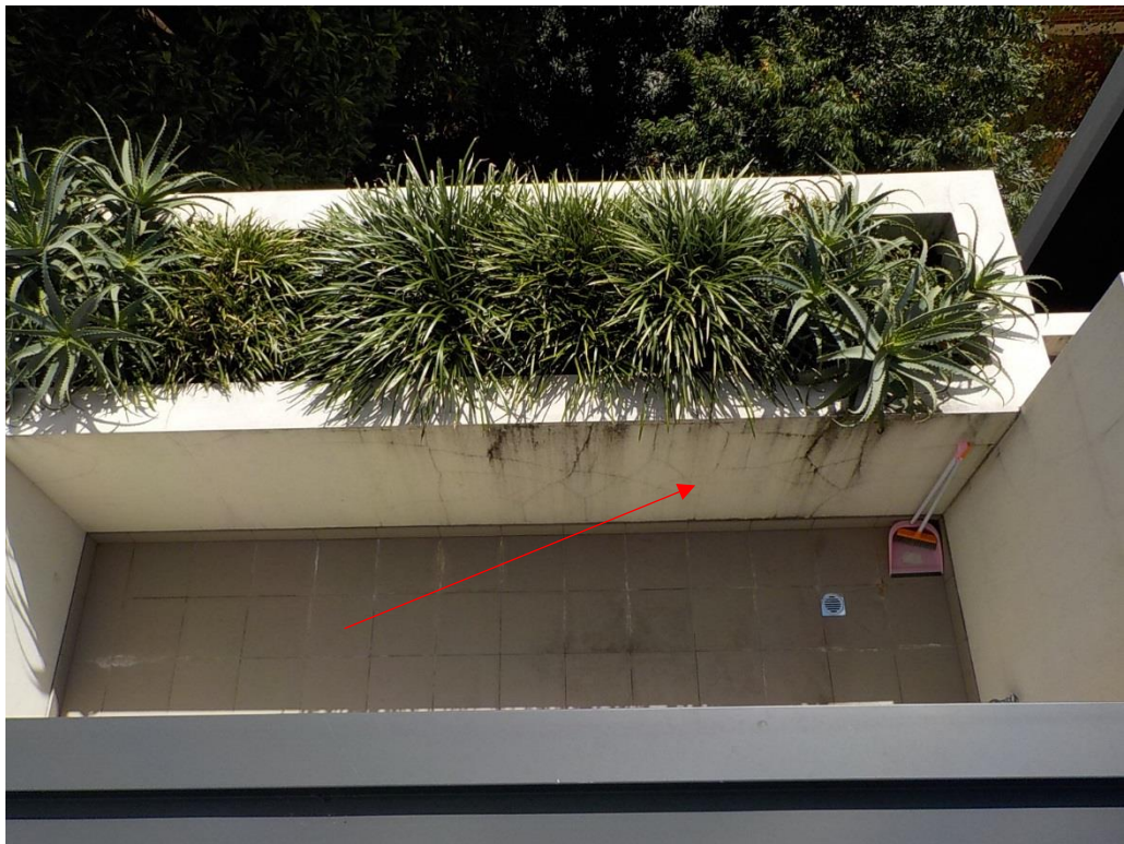
Figure 4 – Unit 18 render repair and façade coating required
