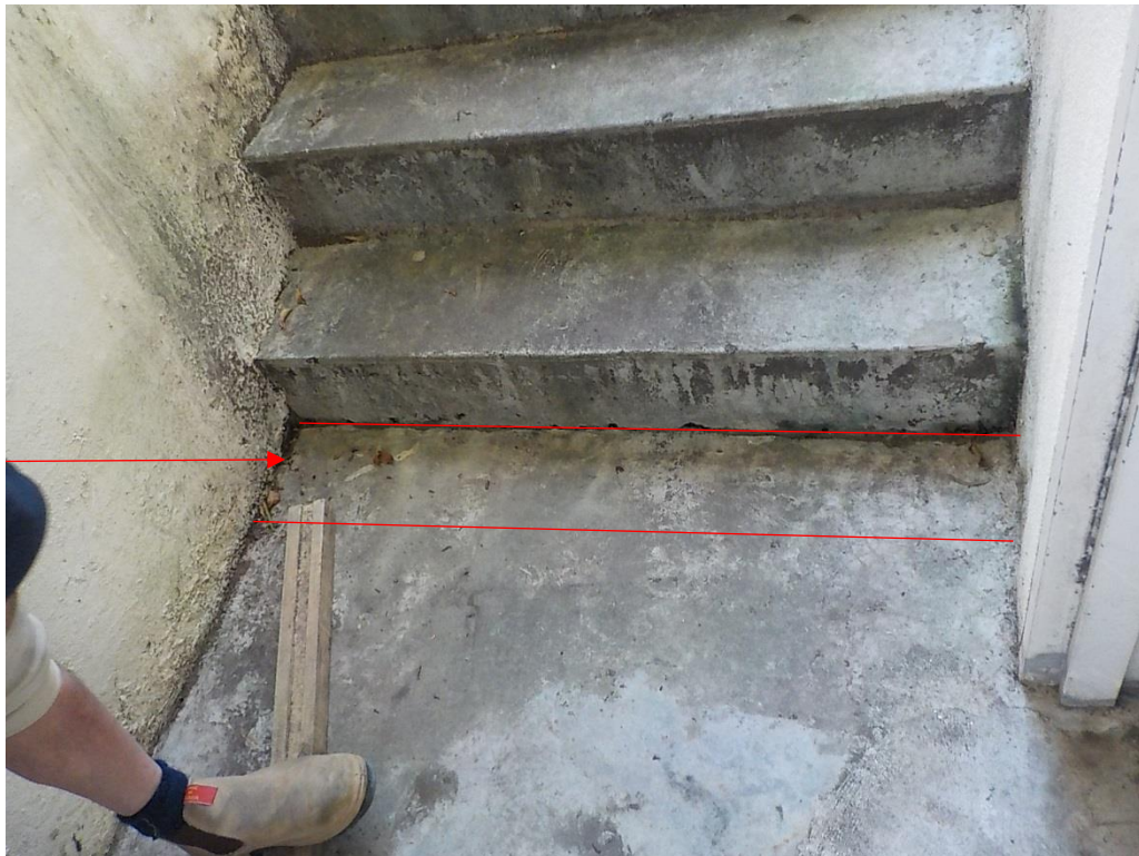
Figure 10 – Fire stair drainage
