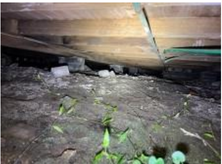
Showing example of low clearances/obstructions preventing reasonable access to parts of the property. Please refer to pre-engagement agreement for reasonable access., (Subfloor)
