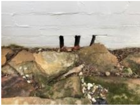
Subfloor air vents are in contact with the ground. Recommend exposing a minimum of 75mm underneath them to reduce the risk of termite attacks/water ingress to the building causing footing and moisture related issues.
