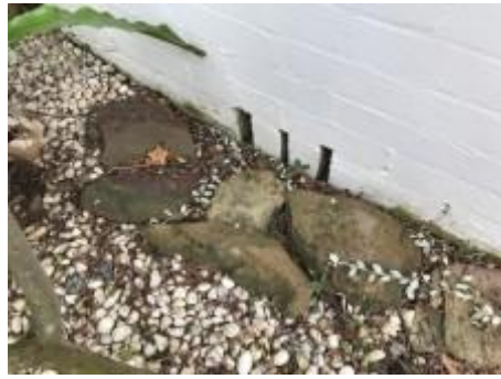
Subfloor air vents are in contact with the ground. Recommend exposing a minimum of 75mm underneath them to reduce the risk of termite attacks/water ingress to the building causing footing and moisture related issues.
