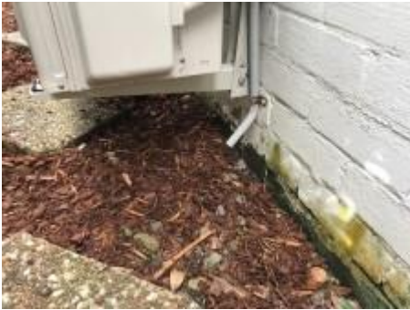
AC unit overflow/s, recommend diverting away from the building or to a suitable drain
