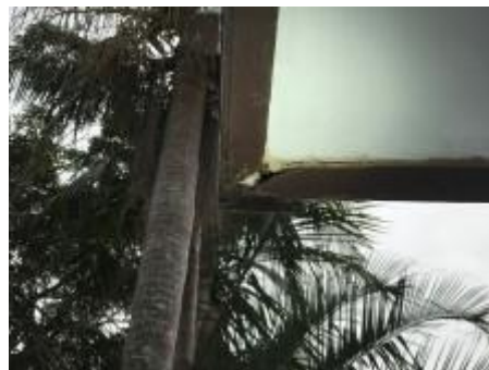
Wood rot to external mouldings
