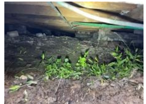
Showing example of low clearances/obstructions preventing reasonable access to parts of the property. Please refer to pre-engagement agreement for reasonable access., (Subfloor)
