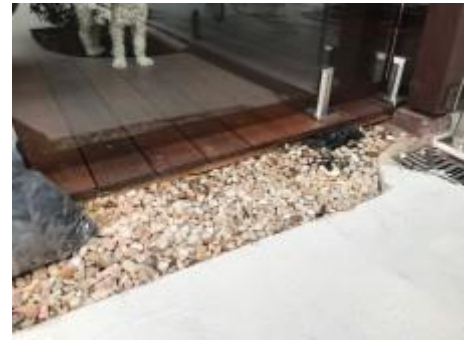
Timber/s in contact with ground - recommend exposing 75mm under timbers to allow for visual inspection zone and to prevent the risk of wood rot and termite attack.
