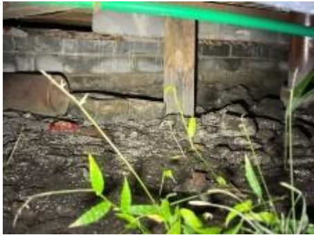
Leaving formwork timbers in direct contact with the ground under a subfloor can significantly increase the risk of termite infestation and structural damage. Termites are drawn to timber, particularly when it is untreated and in contact with soil, as it provides both a food source and a favorable environment for them to thrive. Additionally, the timber can serve as a pathway for termites to access the building. To reduce this risk, any leftover timber in the ground should be promptly removed to eliminate potential food sources for termites.
