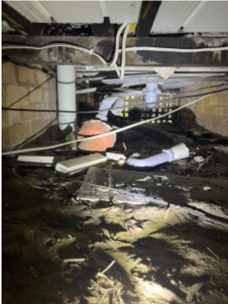
Debris in subfloor
